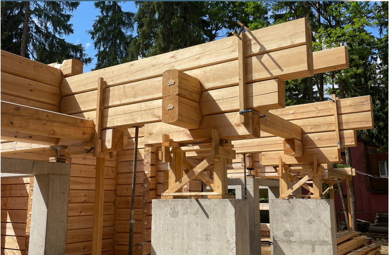
From architectural visualisation to construction — the completed timber log structure assembled on its foundation.
