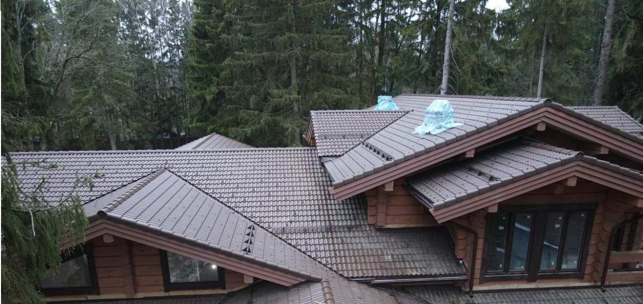
Multi-level engineered roof structure, 800 m 2 Complex multi-level roofing system with a total roof area of approximately 800 m 2 .
