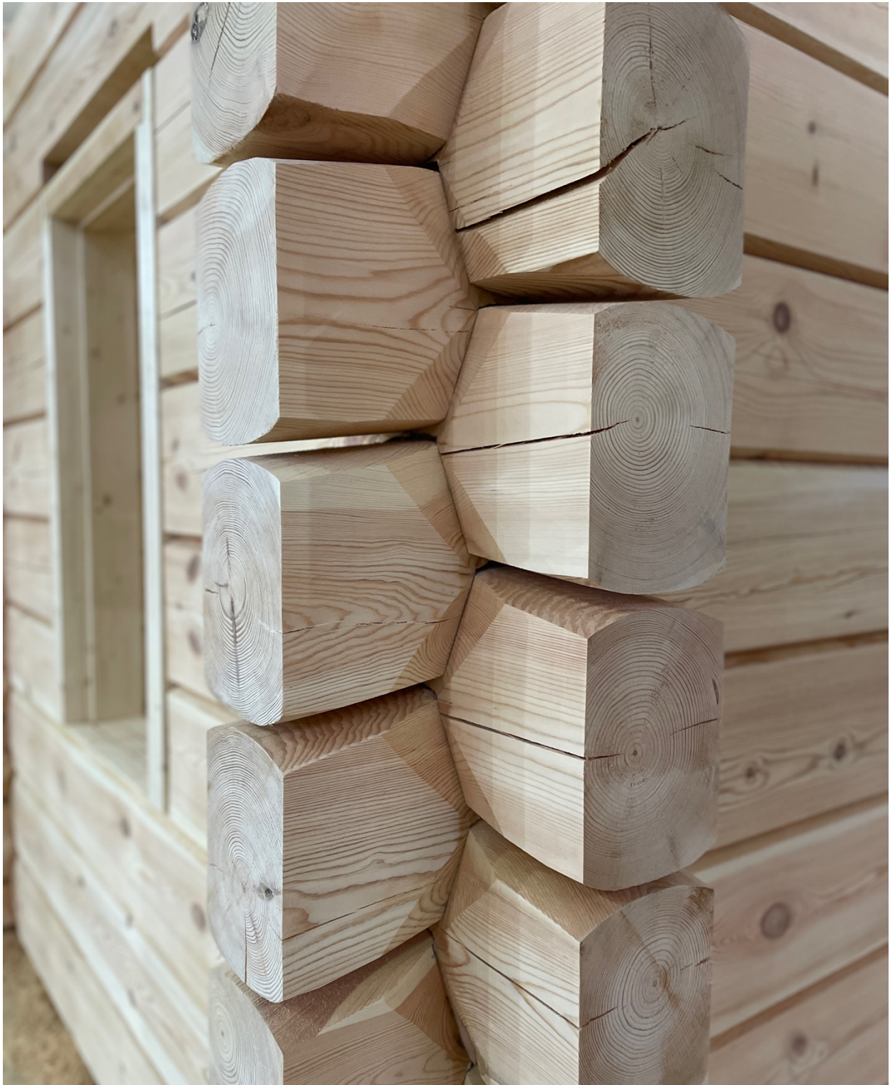
Assembled exterior corner of the log structure Corner detail showing the assembly logic, joint precision, and structural character of the timber wall system.
