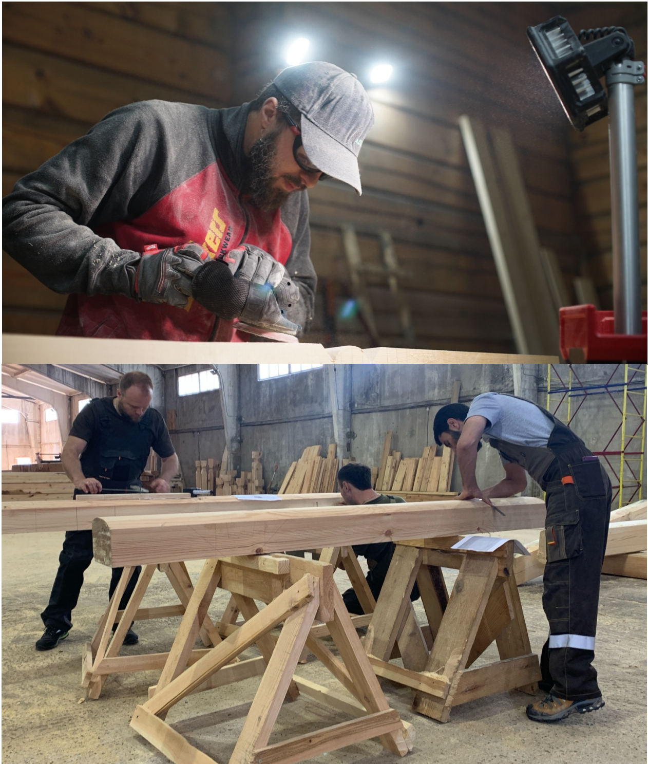
Hand-tool training with kiln-dried timber Participants work with premium kiln-dried timber using traditional hand tools and finely sharpened axes.
