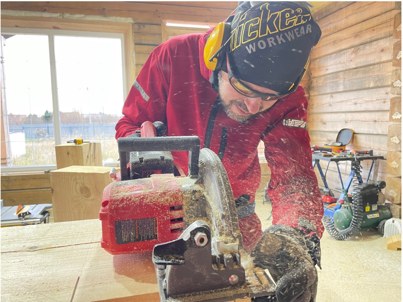
Author at work — preparing structural timber elements for a stavlaft house as part of the workshop-led fabrication process.
